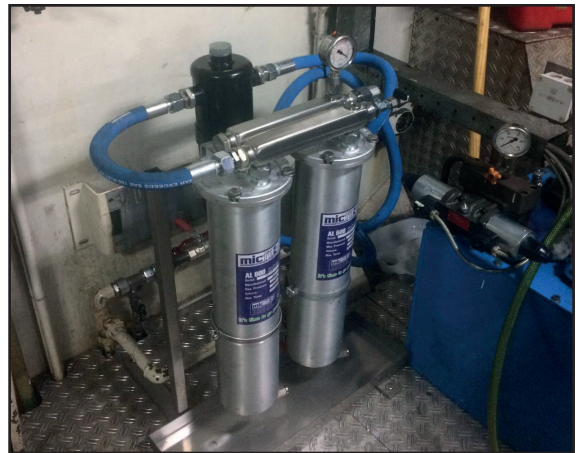
AL600 double system with WS800 for diesel on the main engine
