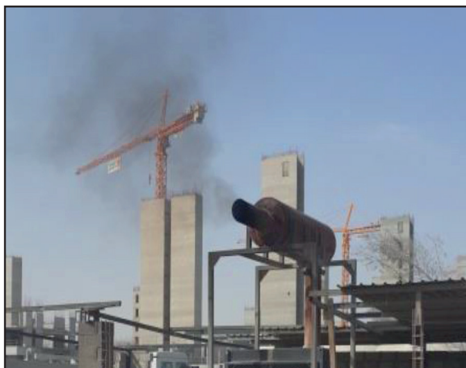
Before the installation of the micfil filters
