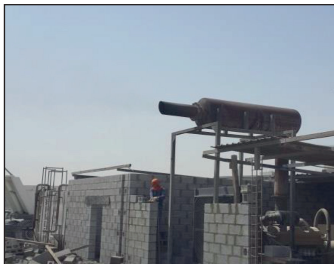
After the installation of the micfil filters
